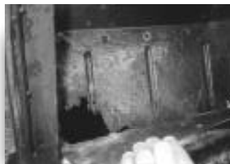
Typical rusted-out hole in the footwell.
